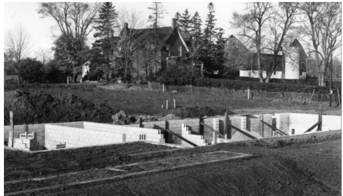
The basement of the new Township Office was being laid out in this Sept. 1962 photo. EHS07884
